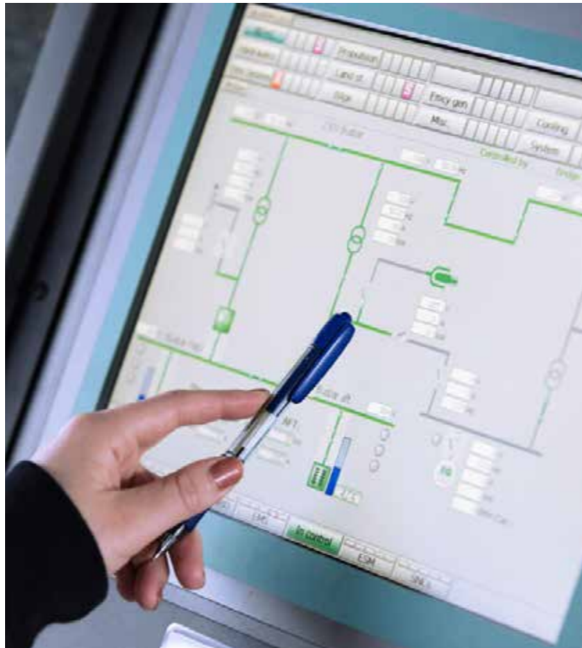
The energy management system (EMS) is pre-programmed with curves giving engine fuel consumption under different load conditions. The EMS interfaces with sub-controllers for gensets, thrusters and remote controls to monitor and set optimal engine speed.
