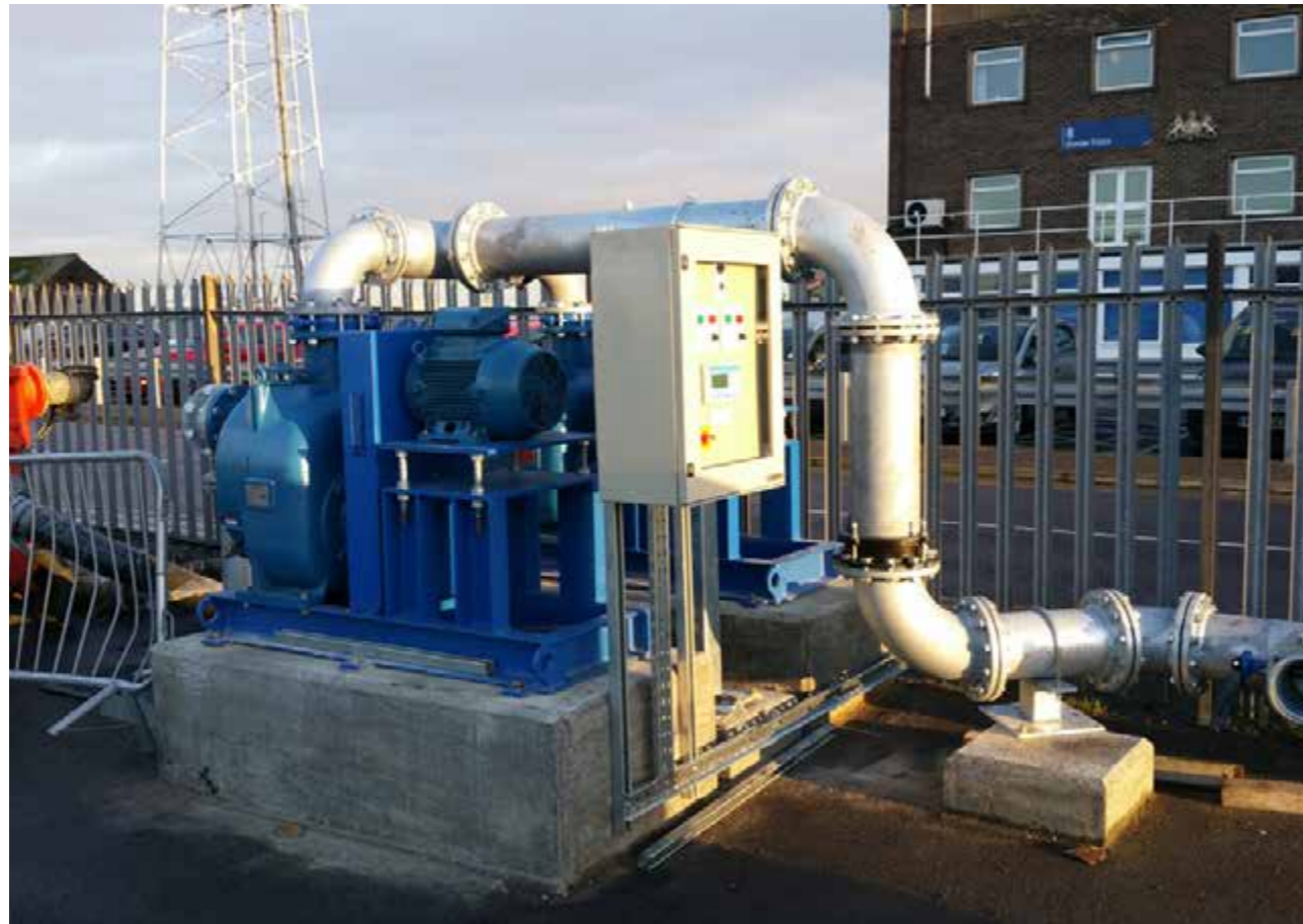
The pumping station is positioned over the discharge pit and comprises of: two Wemco WSP6 self-priming pumps, galvanised Mild Steel pipework, heated jackets for cold weather protection and a control panel c/w pulsar ultrasonic level control.
