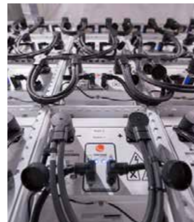
The batteries are charged from hydro power. This battery pack onboard, like the ones on each pier, corresponds to the effect of 1600 standard car batteries. The charging at each pier takes only ten minutes.
