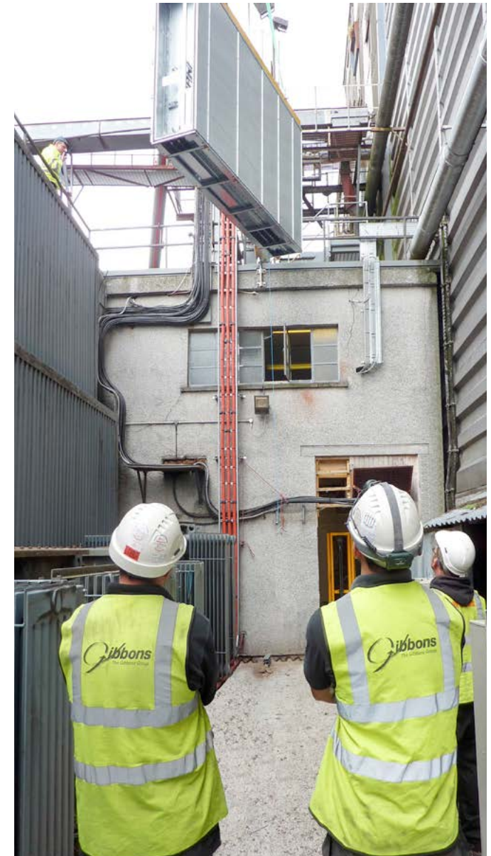
Engineers look on as the drive is carefully lowered towards the plant room entrance
