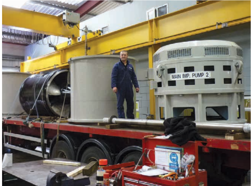
The 40 tonne reconditioned pump and motor back on the low loader heading for Tilbury Docks.
