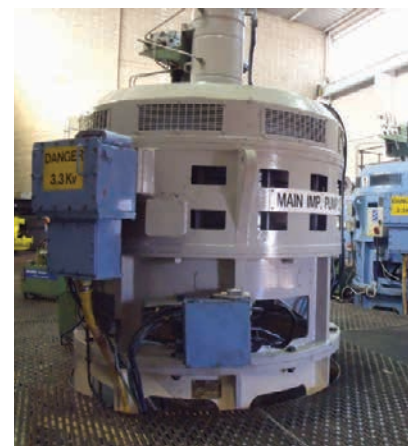
Running smoothly: the reconditioned 50 year old pump manufactured by Armstrong Vickers at their Elswick works in the 1960's.
