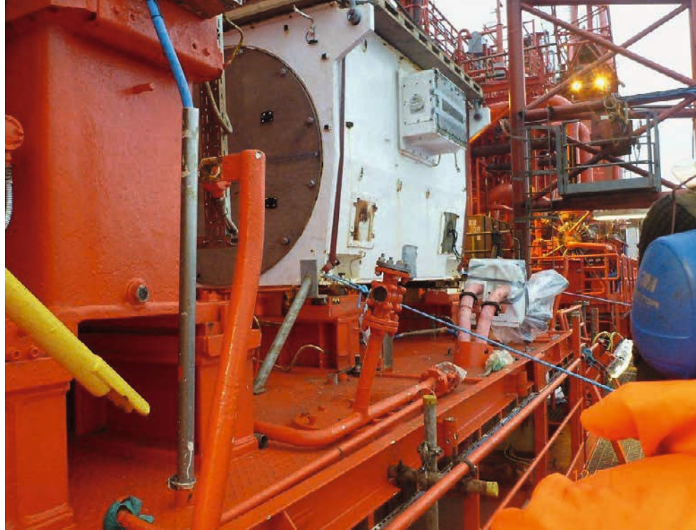
The large High Voltage machine on board the vessel.
