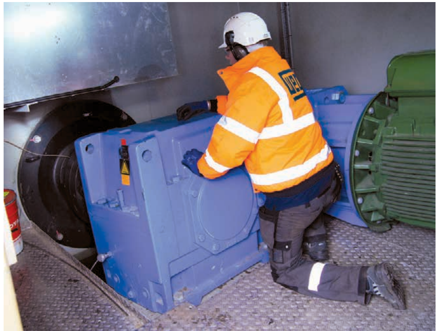
The WEG W22 motor/generator installation and gear box connected to the Archimedes screw.
