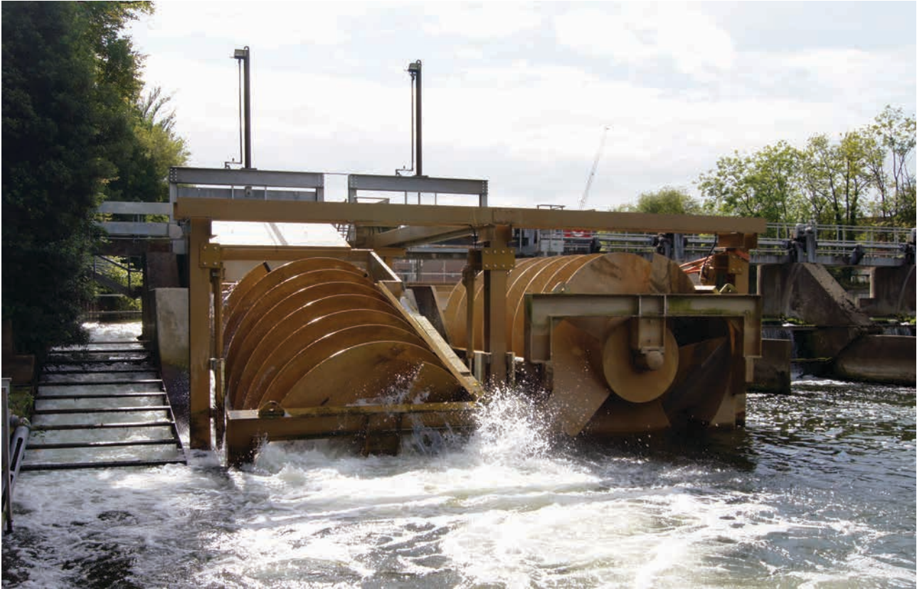
One of the two Archimedes Screw Generators operating at Romney Weir. Next to them on the outside sluice gate is the fish run.
