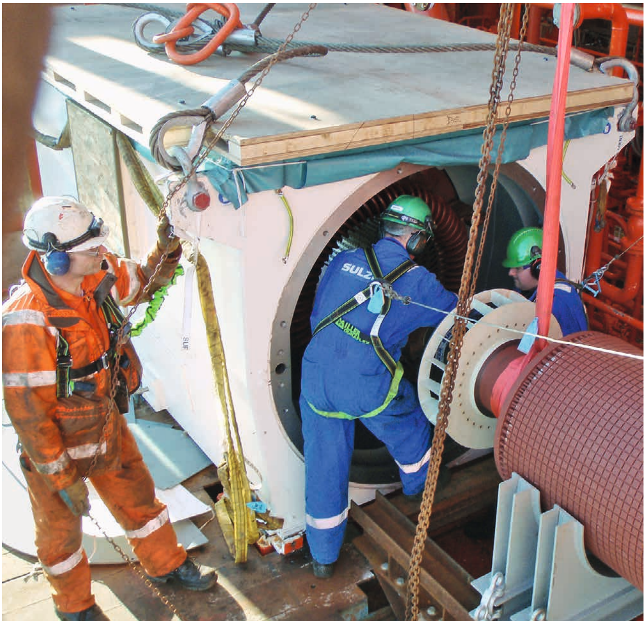
The rotor of the 9 MW machine being removed on board the FPSO in the North Sea by Sulzer engineers, using the special support frame manufactured by their service centre in Falkirk.
