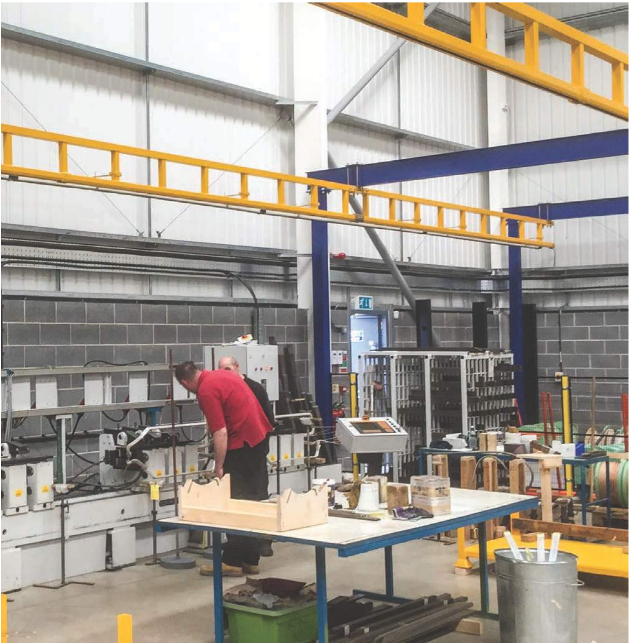
Gantry over the Schumann Hot Coil Press station.
