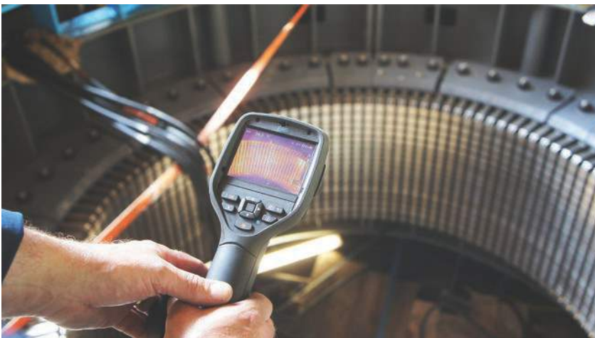
The service team used a thermal imaging scanner to check if the core laminations had a uniform temperature spread.
