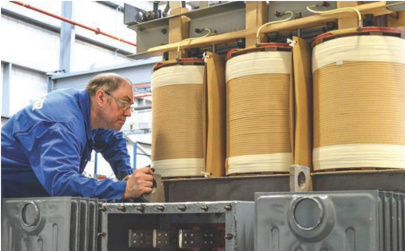
Sulzer was recently contracted to complete the refurbishment of a transformer for Redcar Bulk Terminal.
