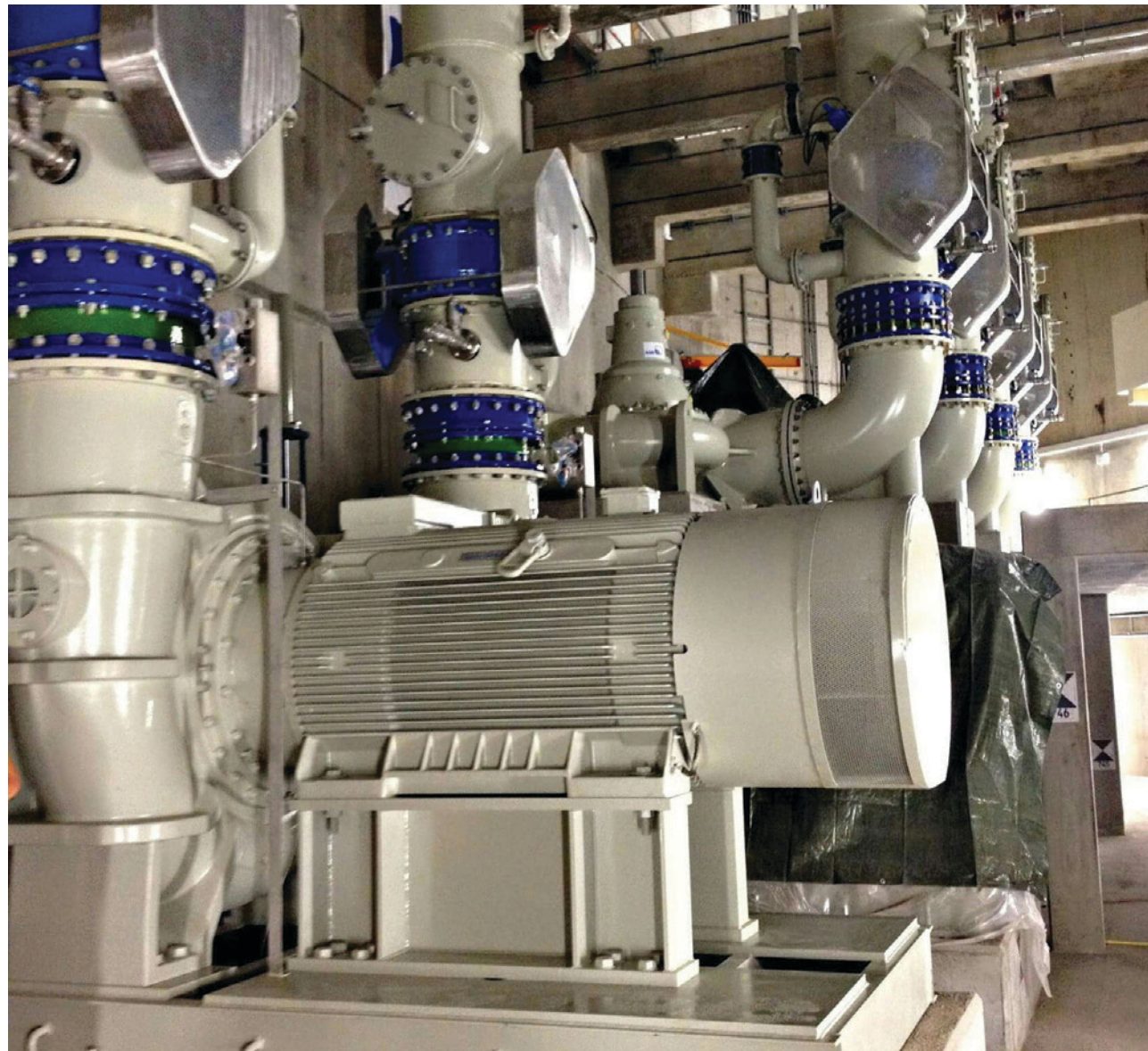
KSB Sewatec Pumps for Europe's Largest Wastewater Project at Emscher Sewer Canal Pumping Stations Germany
