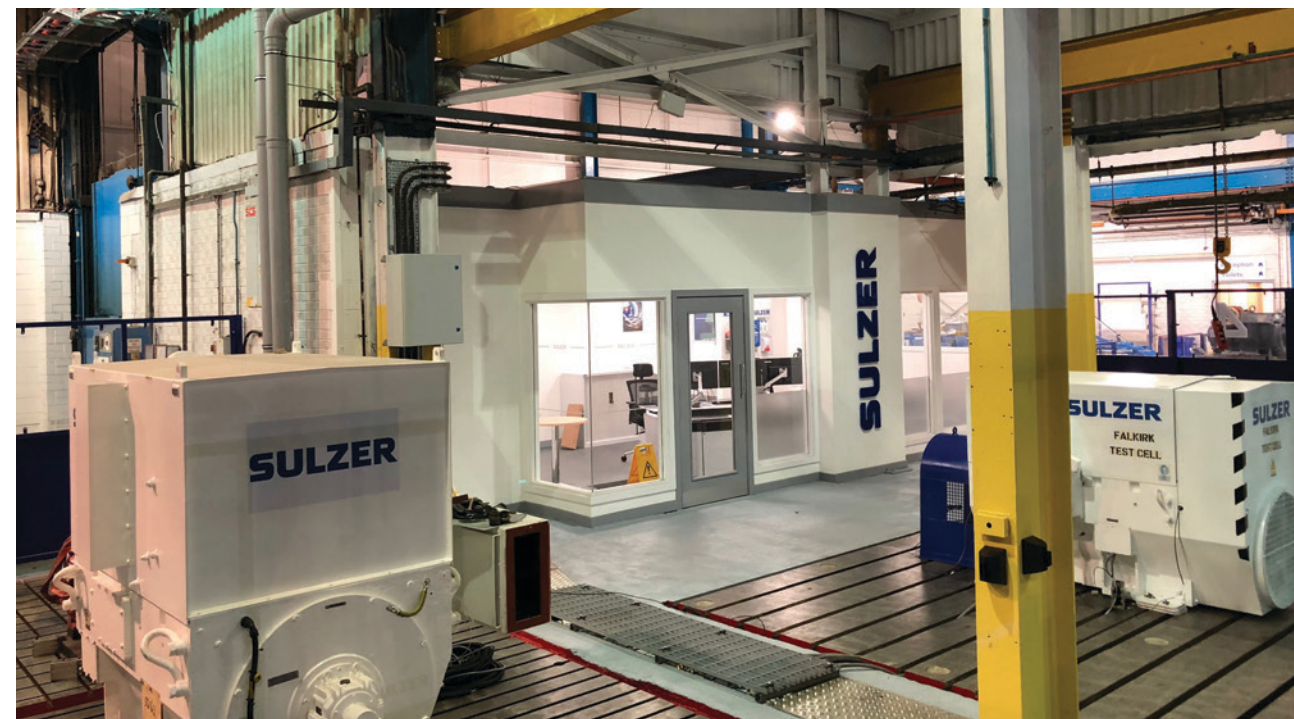
The new installation increases the load testing capacity to 2,000 kW for horizontally-orientated motors as well an increase in voltage to 13.8 kV.
