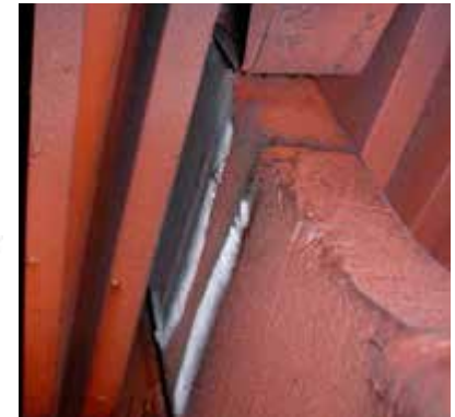
Damage by PD
